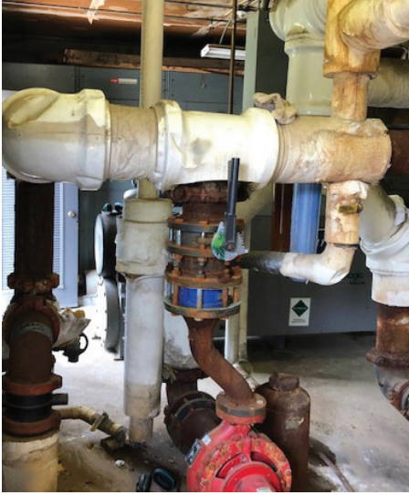
A complete repipe from the mechanical room to the fan coil units was long overdue.
